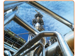
Chemical, Oil and Gas
